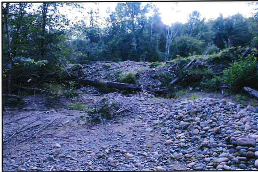
Figure 19. Entrance to low-flow side channel blocked by berm at Bennett Site.
