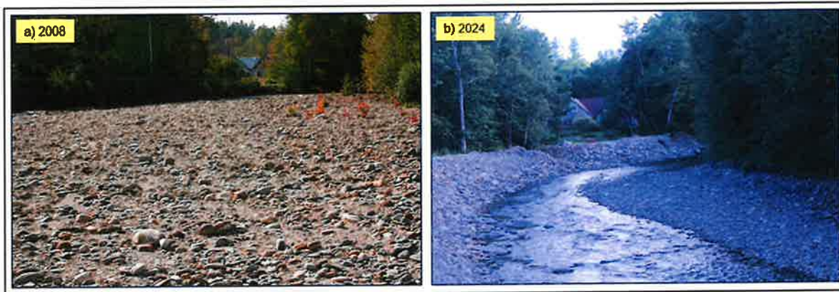
Figure 16. Photos from the same location looking upstream at the Rollins Site in a) 2008 and b) 2024 showing how large cobble point bar was excavated to form new channel and adjacent “in channel” berm.
